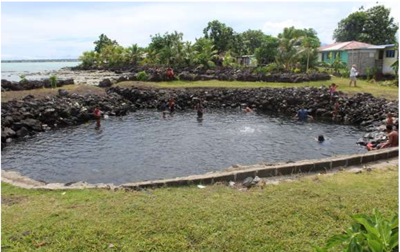
Vaitoomuli coastal spring pool use as back-up water supply for bathing. The rock-wall surrounding the pool is eroding. Photo credit: MNRE-PUMA, 2017
