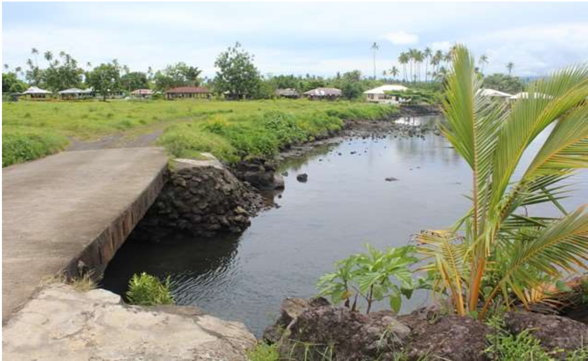
Old Cement Bridge Vailoa village access to the old village on the coast, potential high risk as the bottom is eroding and unstable. Located in the coastal hazard and flooding zone Photo credit: MNRE-PUMA, 2017
