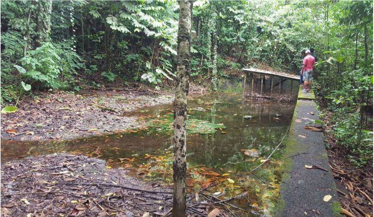
Old water reservoir inland of Tuanai village build during the German times (according to village mayor) village representatives expressed the need to rehabilitate the reservoir as an alternative option to support inland families without access to water.
