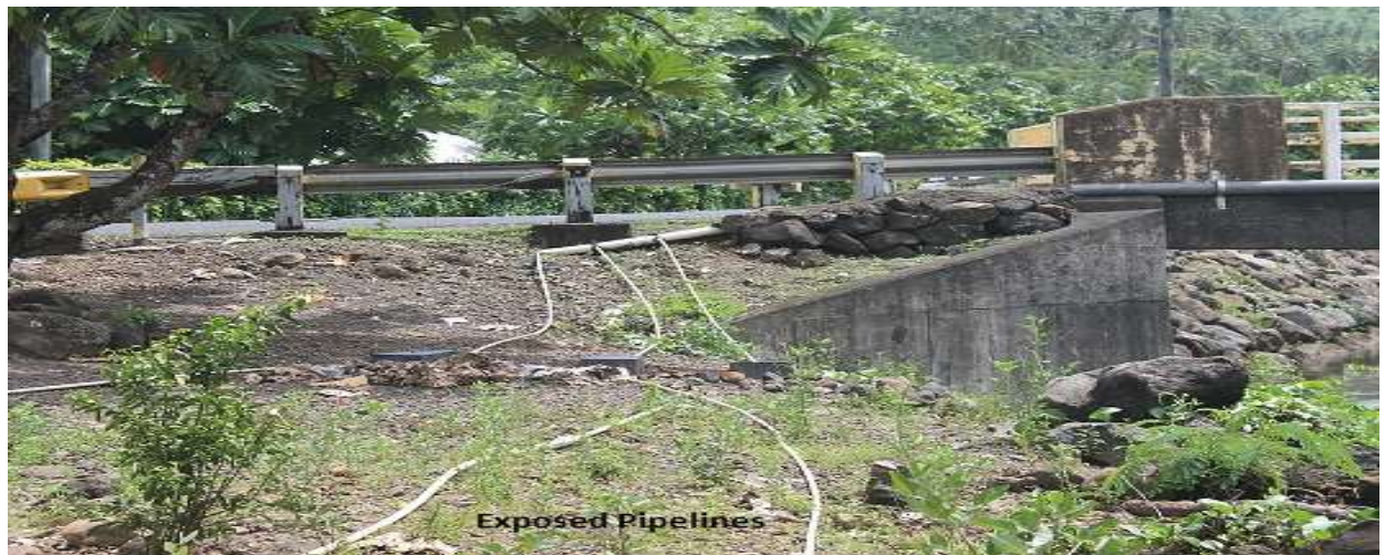
Poorly drain access road
