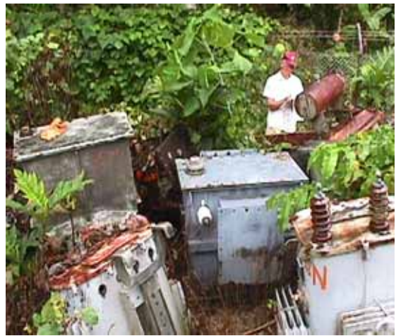
4. Transformers including PCB-contaminated at Electric Power Corporation, Vaitele. GoS, MNRE (2003)
