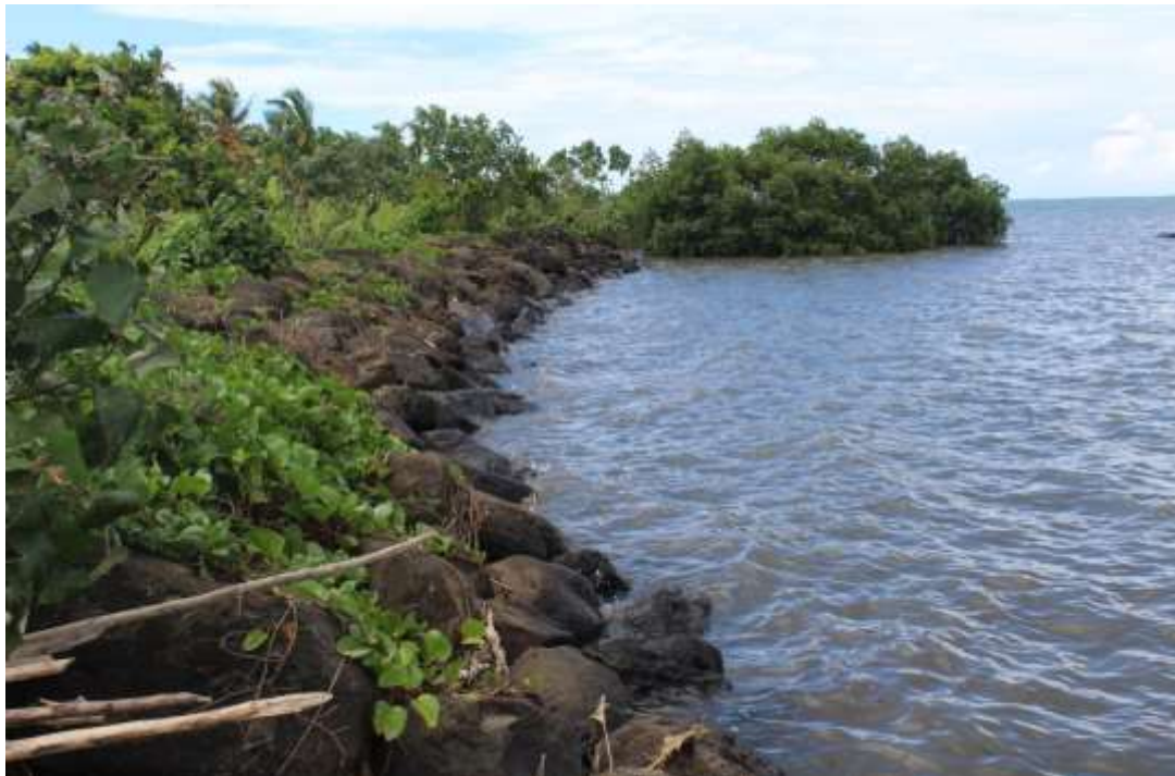
Rock revetment at Vaigaga coastal area – loose rocks starting to fall out from strong waves and sea-level rise
